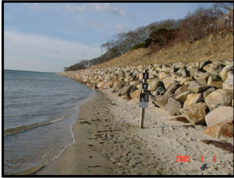
The loss of public lateral beach access due to shoreline armoring along the shore of Chatham, Massachusetts. Prior to revetment construction, a dry sandy beach provided lateral public beach access to a U.S. Fish and Wildlife property. Photo O’Connell, USGS.
