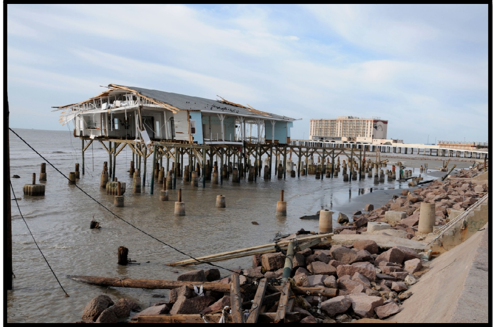
Storm surge damage from Hurricane Ike in Galveston, TX (2008). There were once 4 piered structures along this section of the seawall. Photo: NOAA Flower Garden National Marine Sanctuary.
